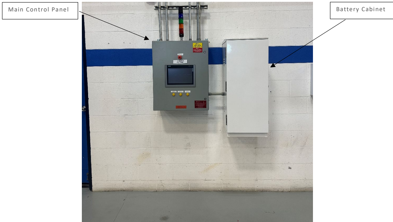
Figure 13-3: Battery cabinet mounted on wall near main control panel
