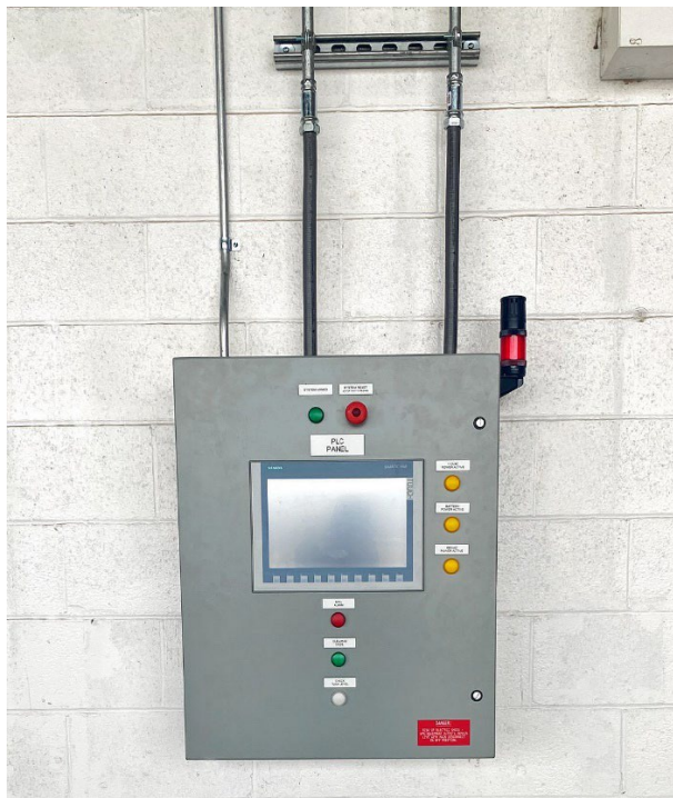
Figure 13-1: ILDFA Control Panel mounted on the interior hangar wall
