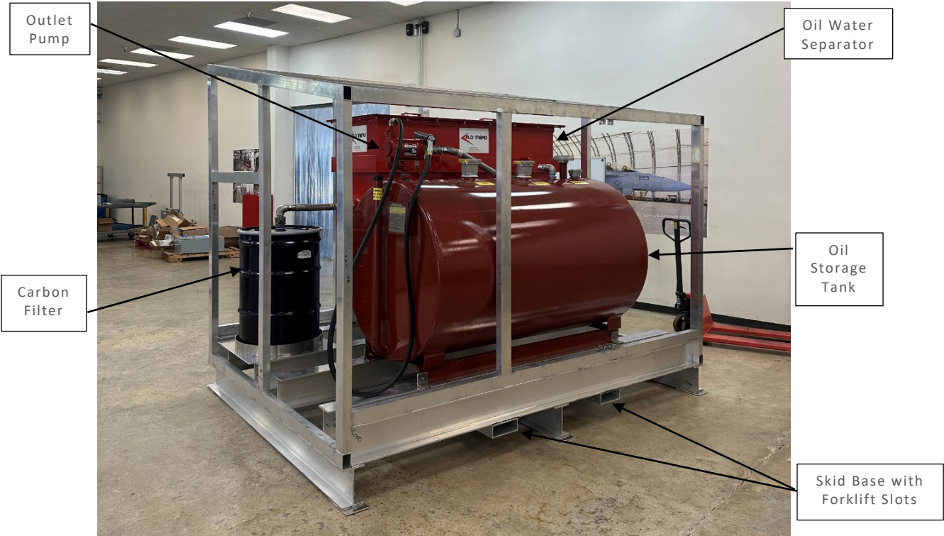
Figure 16-3: OWS Skid Internal (panels removed)
